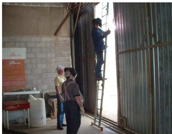
Jim Snelgrove & Loren Henson watch Gray Bridwell weld gap seals on the hangar doors.
